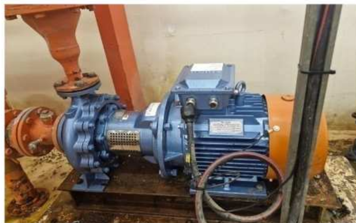
Pump set after
