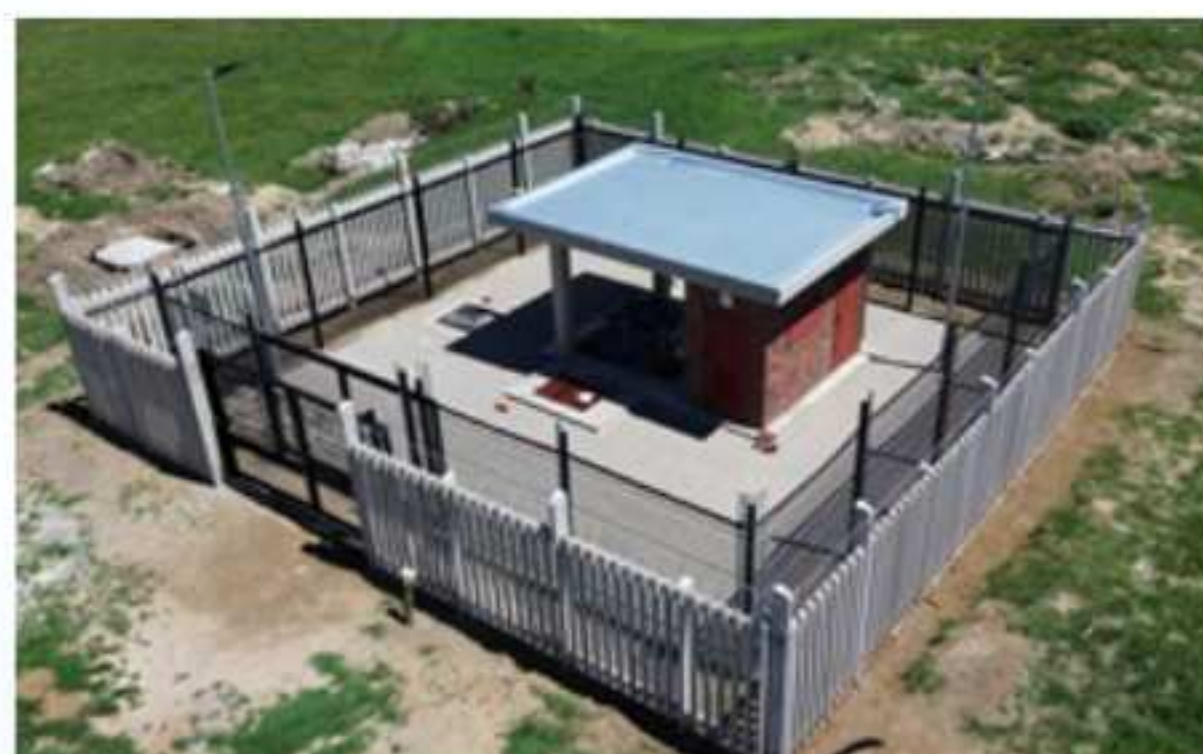
Bronville North Pump Station (Thabong)
