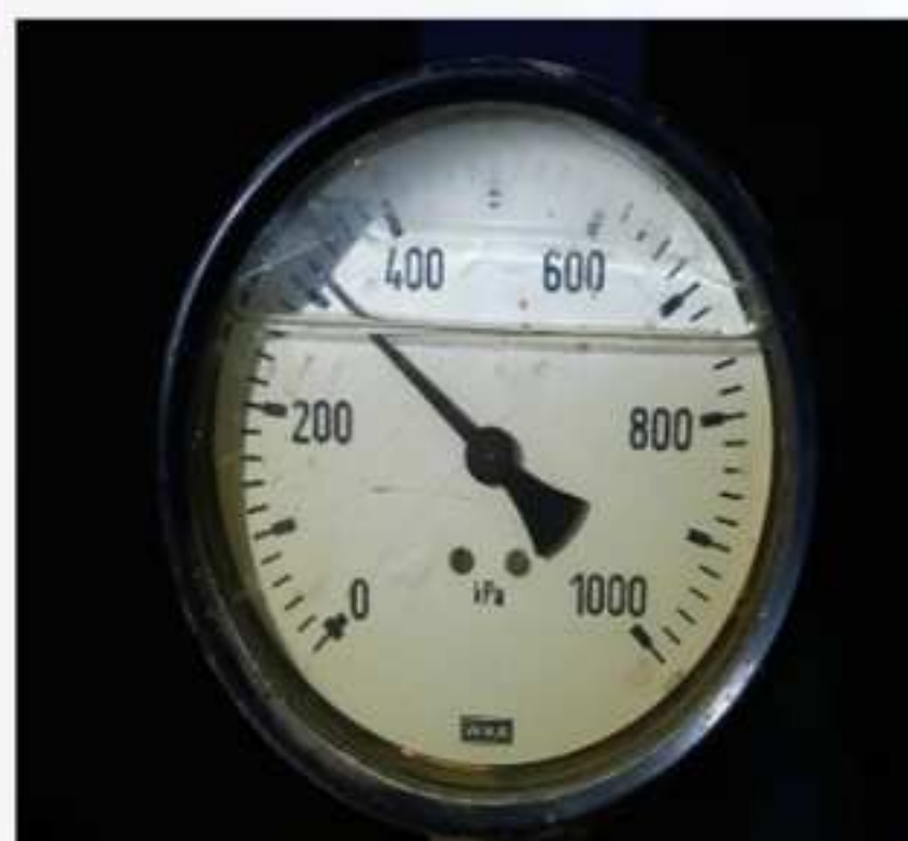
Water pressure gauge indicating sufficient pressure to supply TMDM
