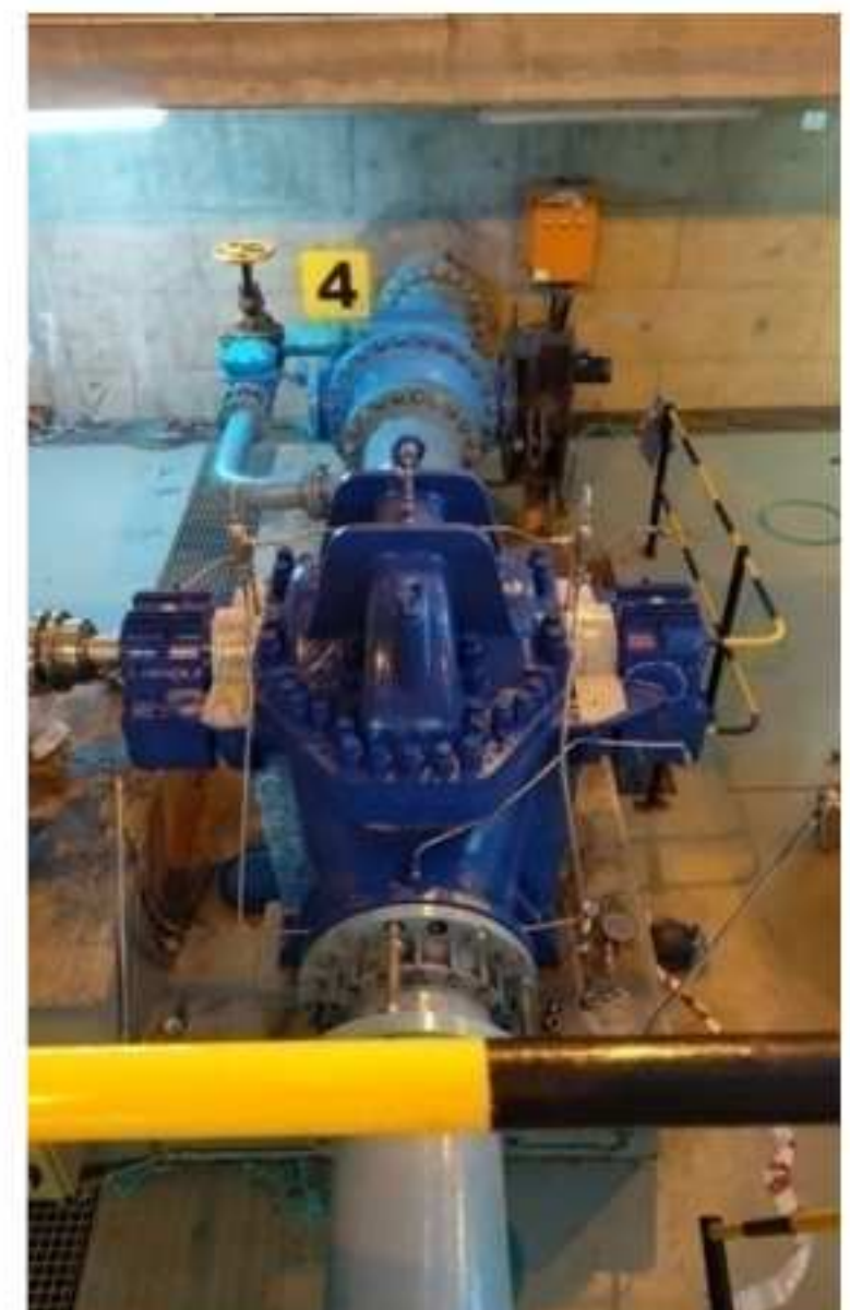
Refurbished Secondary Pump 4
