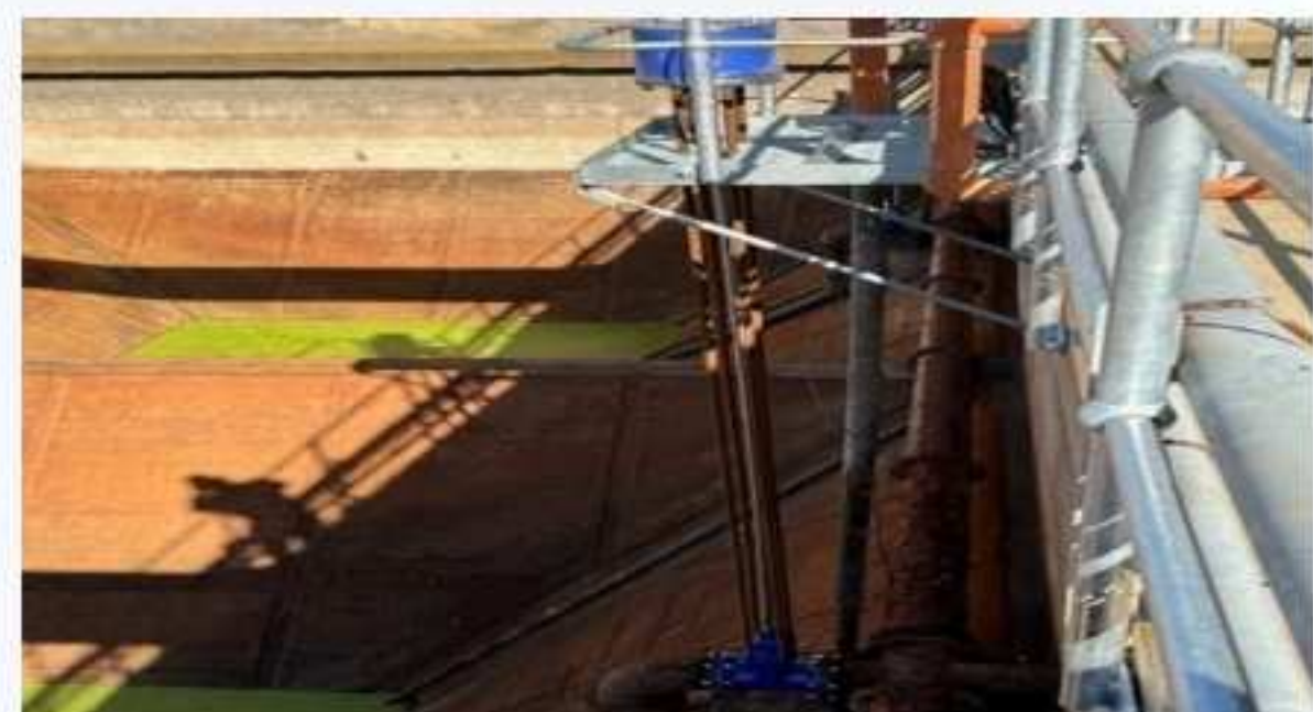
Installed valves and actuators
