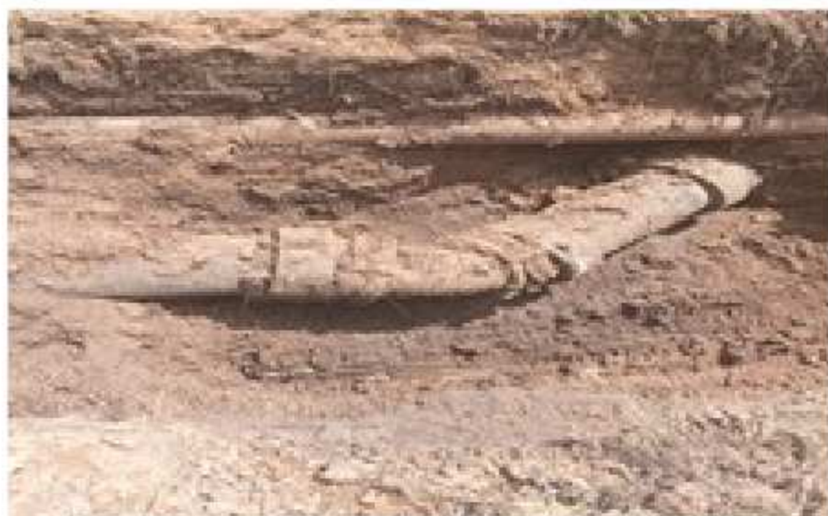
350 mm pipe burst on elbow section
