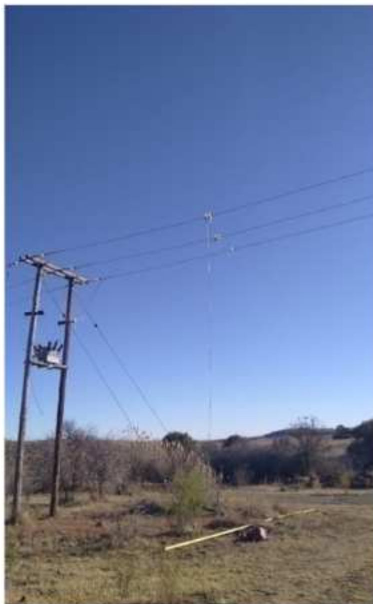
Vandalized 22 kV electrical cable
