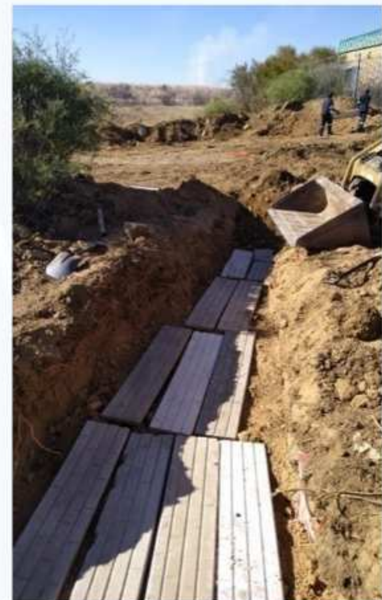
Secured cable avoiding vandalism
