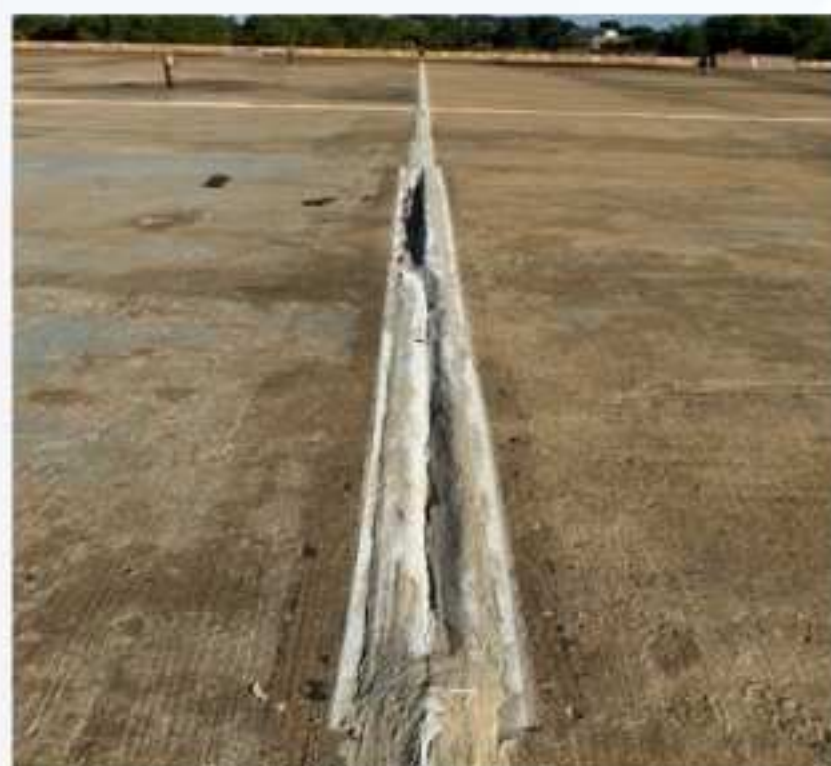
Damage expansion joints on the Allanridge Reservoir
