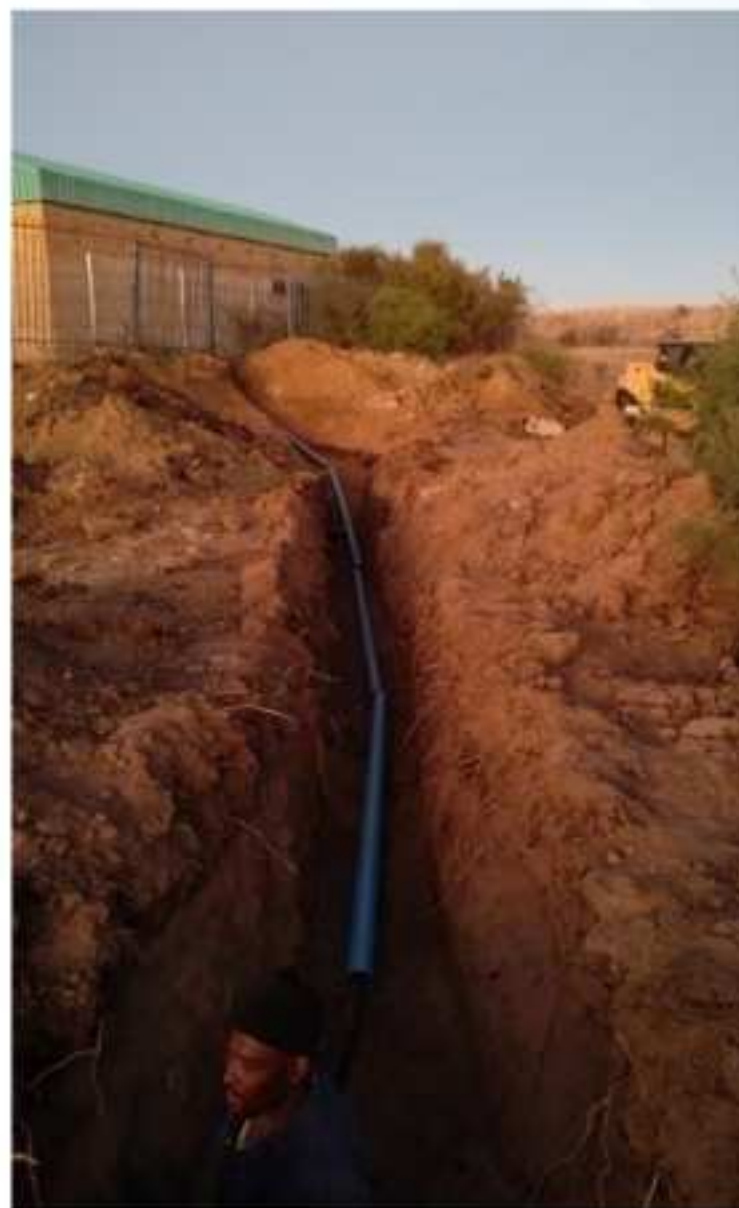
Laid sleeved electrical cable
