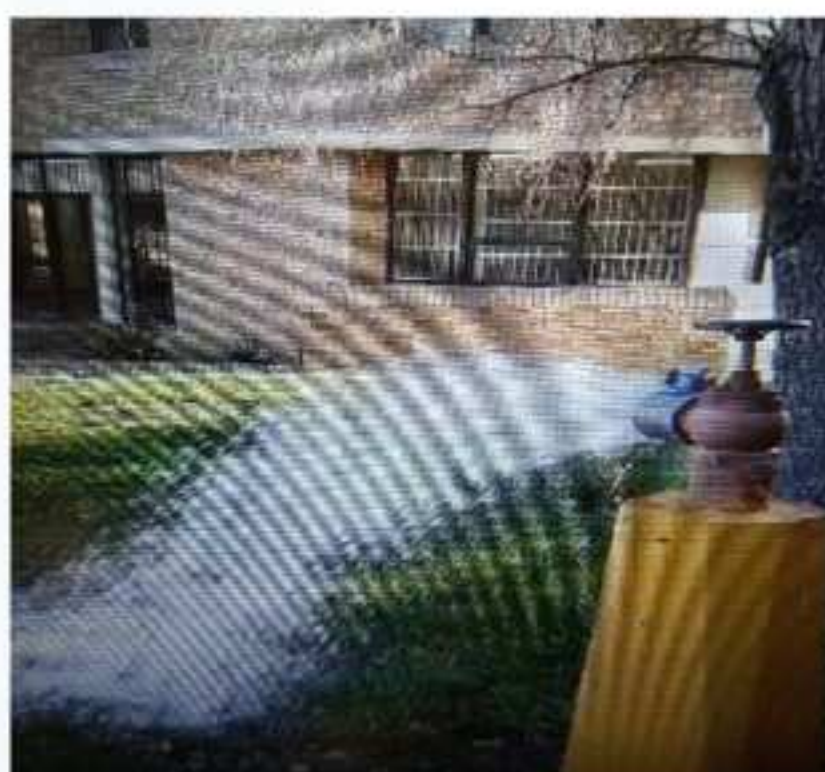
Fire hydrant is displaying sufficient pressure
