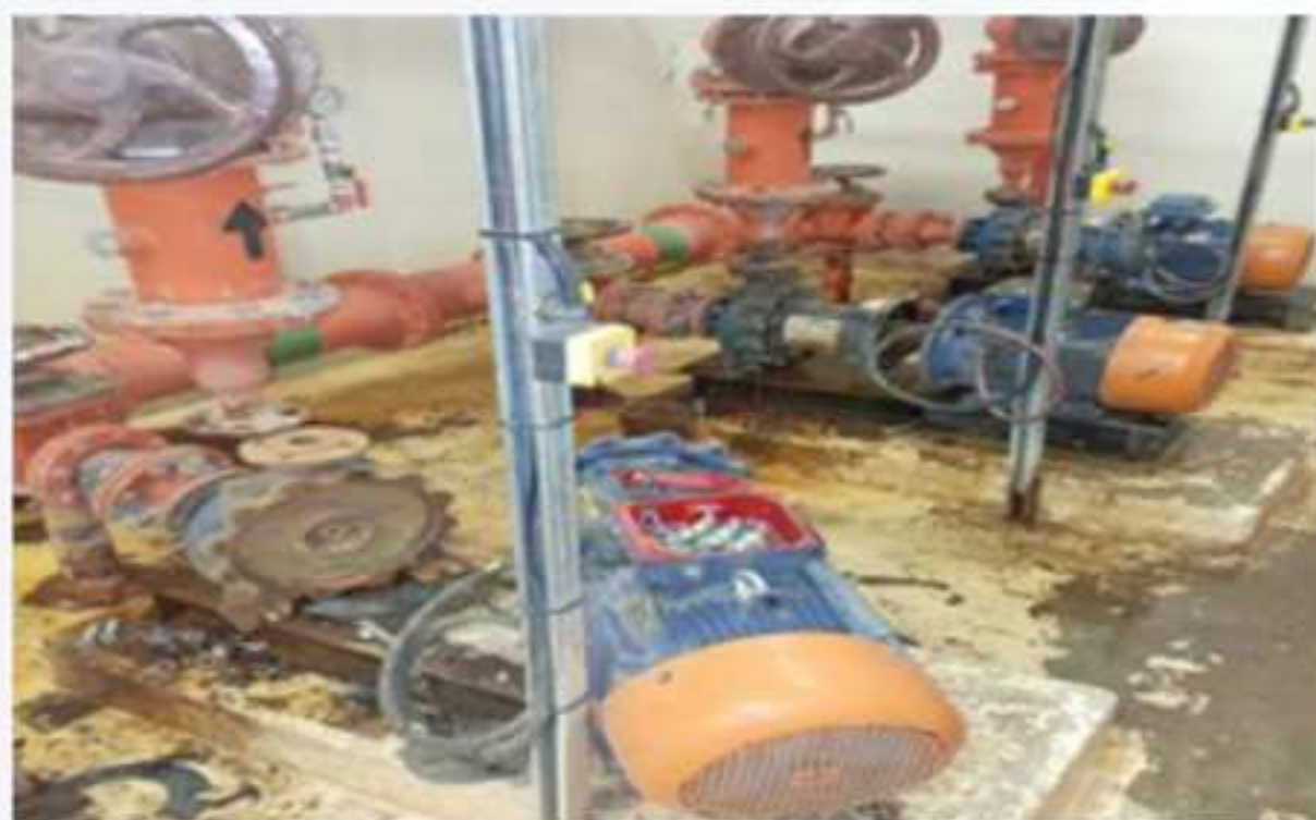
Pump set before
