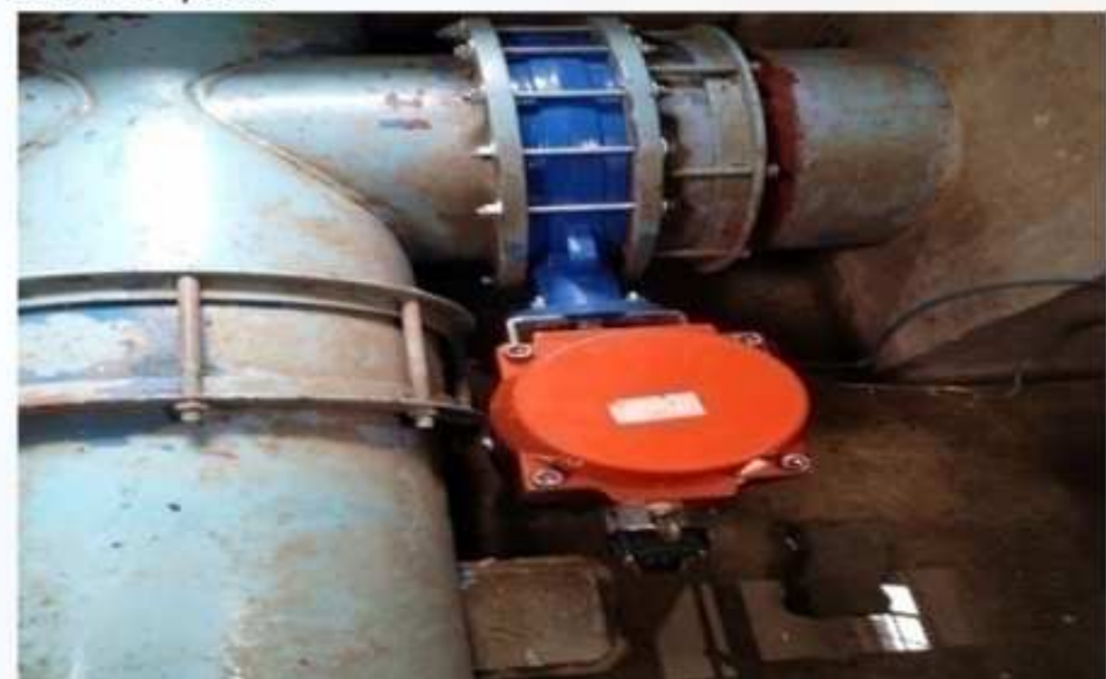
Actuated air release valves
